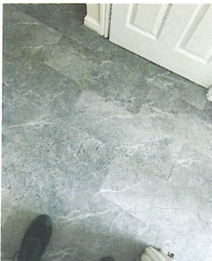
This floor had a lot of movement underfoot when walked over, which was caused by an uneven subfloor and use of additional (laminated) underlay. After a period of just 5 months, the floor had broken on many joints due to stress on the joints of the click system.
